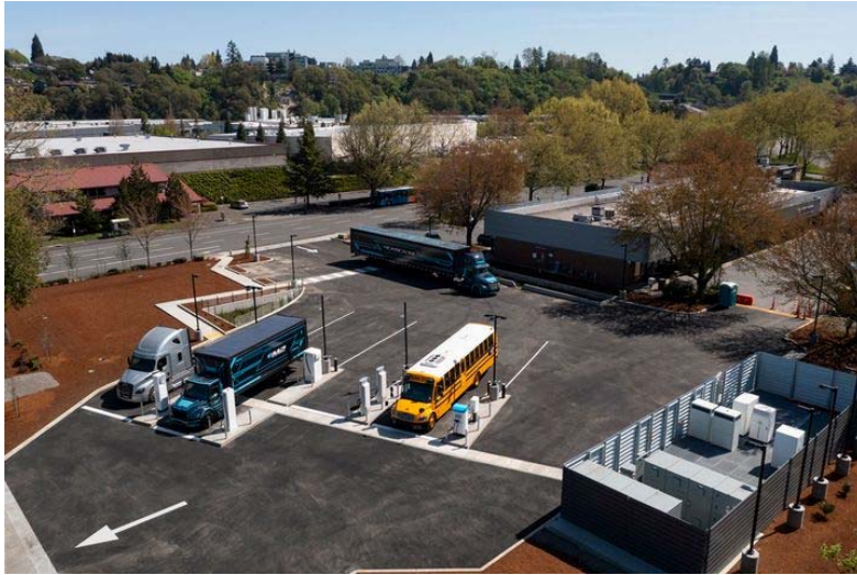
Figure E.4 Electric Island, Heavy-Duty Electric Charging Station in Swan Island, Portland
