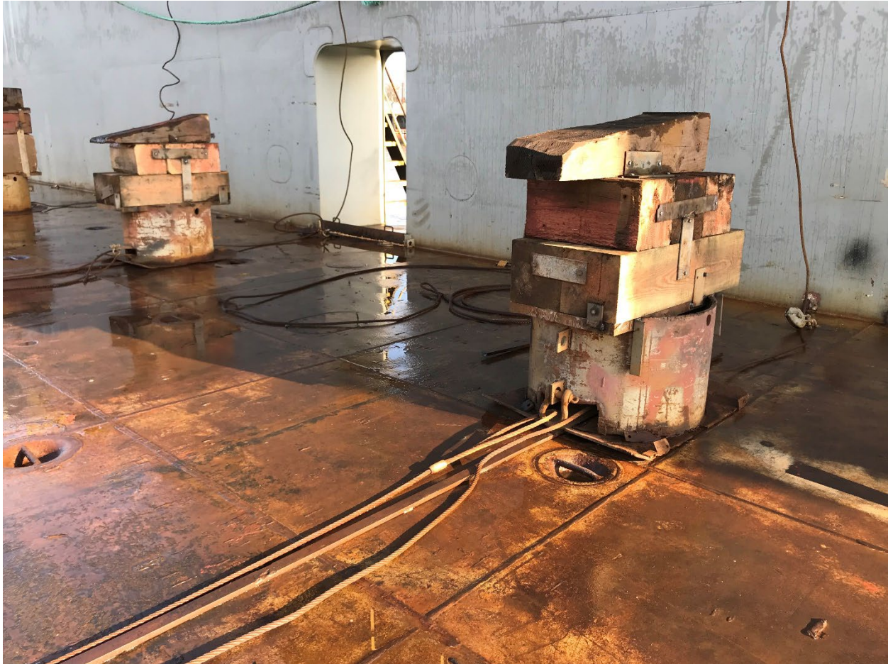
DD-2 Drydock Floor has been shoveled, broomed, washed and all waste collected – no residuals.
