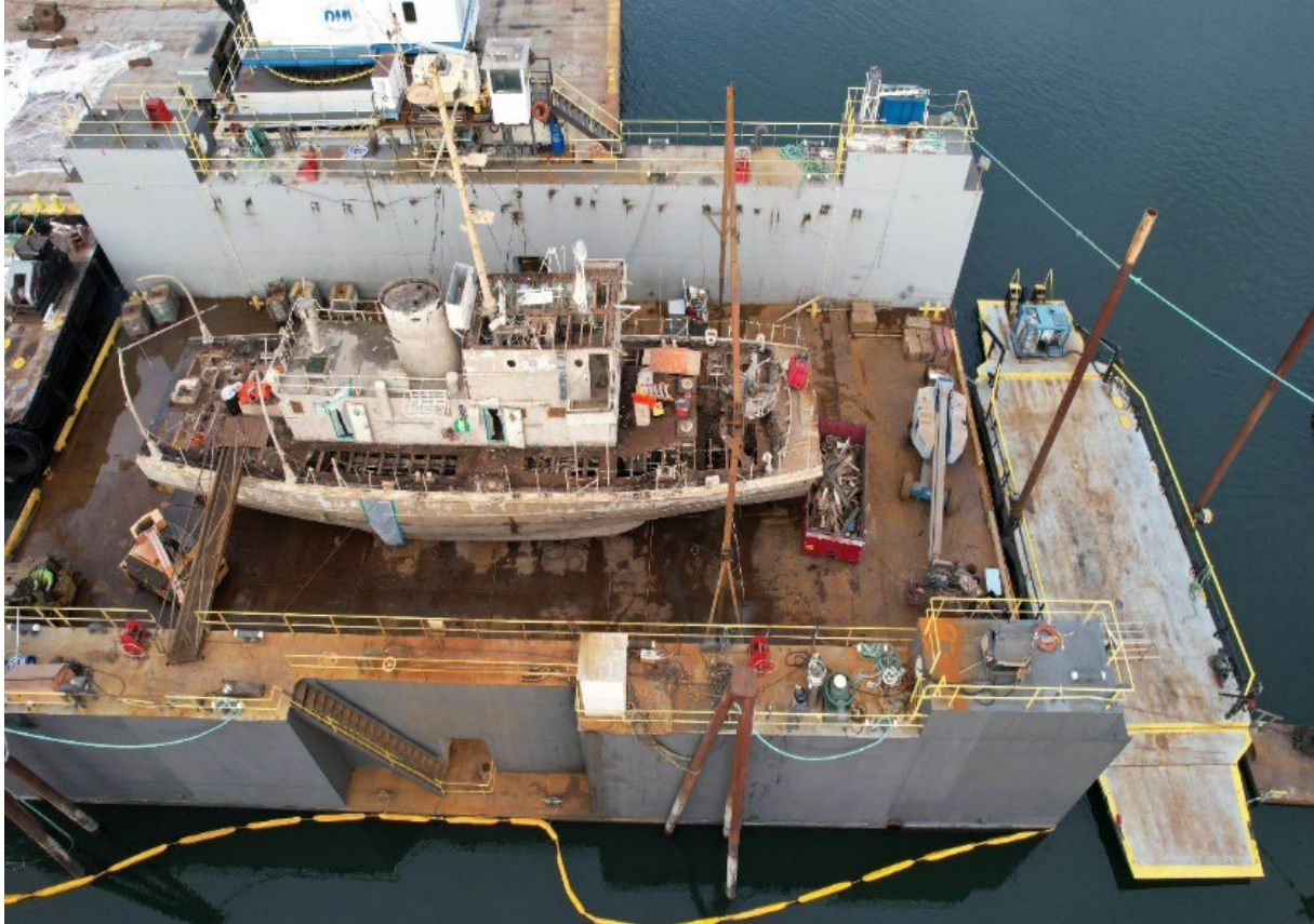
Alert – Vessel in DMI Drydock No. 2 – Bow & Stern Cuts completed with Sections Removed to Barge
