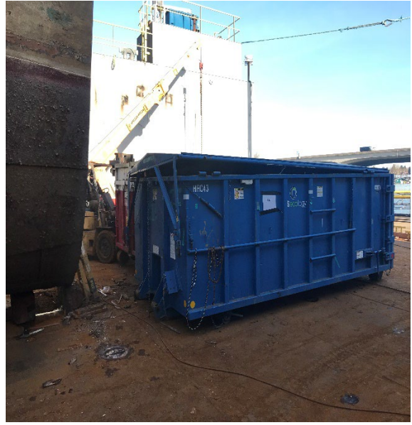
Blue 20-Yard Closed Lid Container for PCB-Lead Bags
