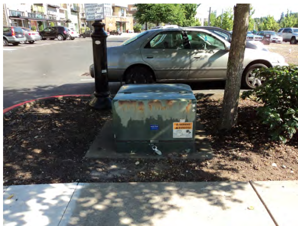
Photo #6 View of a non-PCB labeled pad-mounted transformer located near the southwestern corner of the Property.
